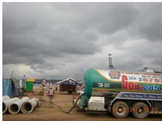
Figure 4.2 Sanitation water of workers on the construction site is collected and treated in accordance with regulations
