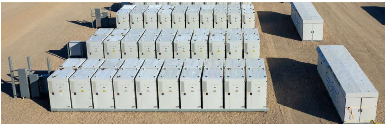
Figure 3-4. Example of BESS compound
