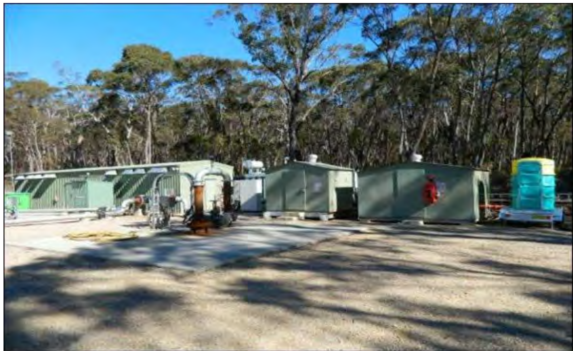
Photograph 3.1: Typical Dewatering Facility
